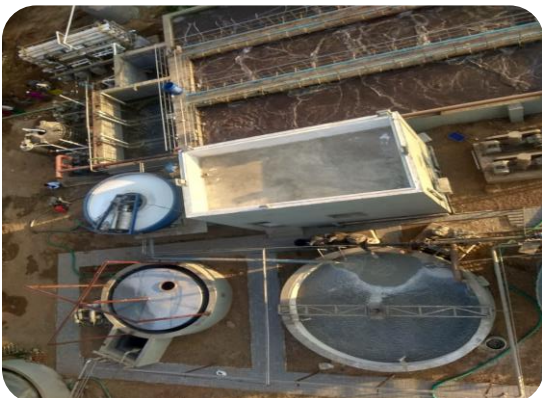
ICR+MBR based Effluent Treatment Plant
