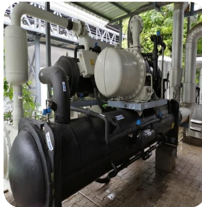
Package Chiller Compressor
